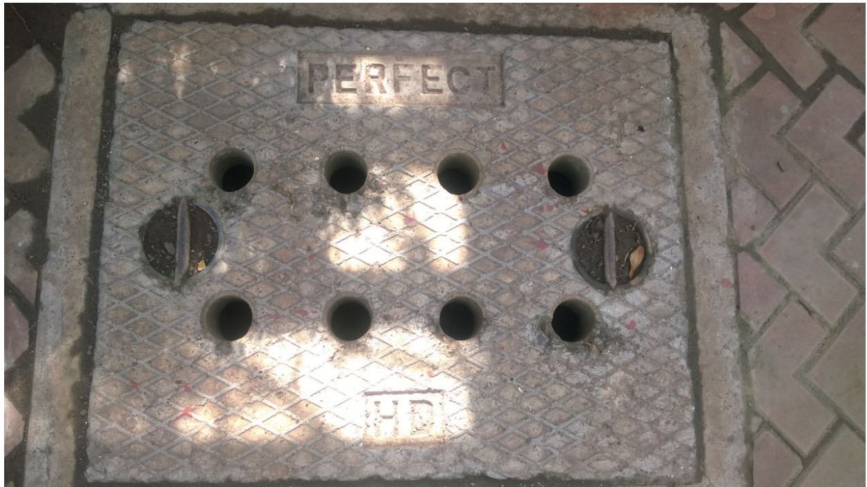
Rain Water System
